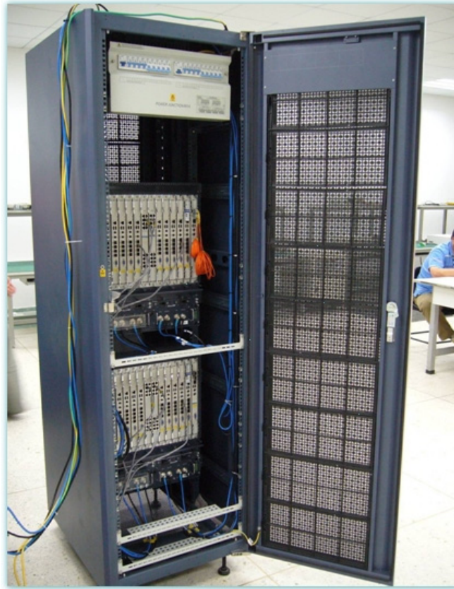
Figure 4: An Overview of a Blade System with the Back Door Open
